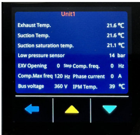
Status screen 1 – refrigerant circuit and inverter
