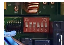
DIP switch block SW1–SW6 on the control board
